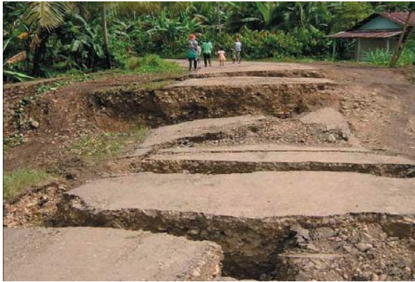
Figure 7. Cracks on an Unpaved Road due to Lateral Spreading, March 28 Nias & Simeulue Earthquake [11]
