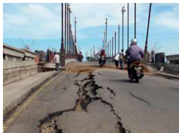
Figure 6. Damage Caused to an Approaching Ramp to Siti Nurbaya Bridge [13]
