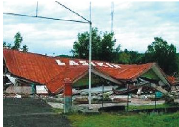
Figure 5. Collapsed Airport Terminal Building in Simeulue [11]
