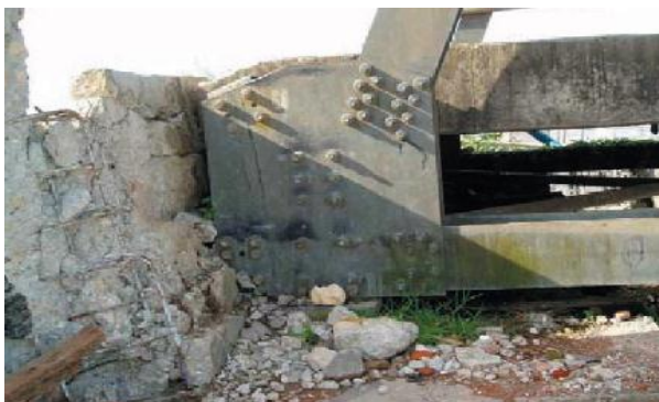
Figure 4. Displaced End Support of a Bridge in Nias [11]
