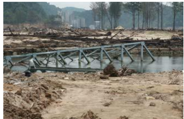
Figure 11. Steel Truss Bridge Swept off its Supports during the Aceh Earthquake [16]
