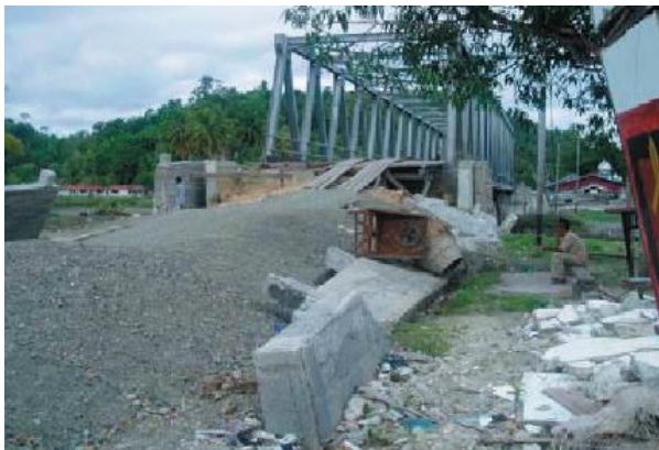
Figure 9. Settlement of a Bridge Approach in Simeulue [11]
