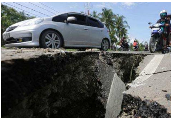
Figure 8. Cracks on the Road due to 2016 Pidie Jaya Earthquake [14]
