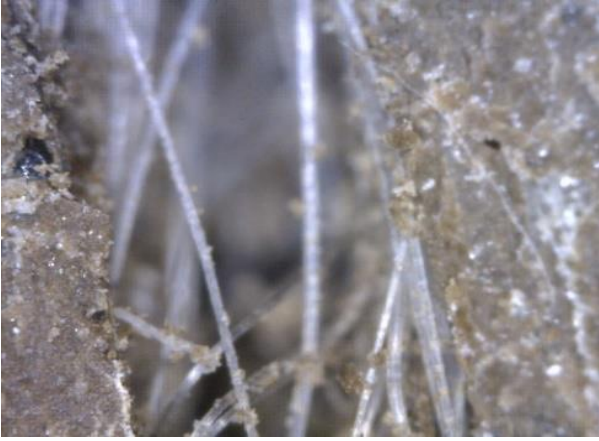
Figure 10. Fiber is Alongside the Crack Direction (750x magnification)
