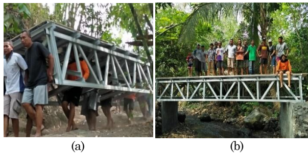
Figure 10. People carried the bridge model (a) and final location of the bridge model (b)
