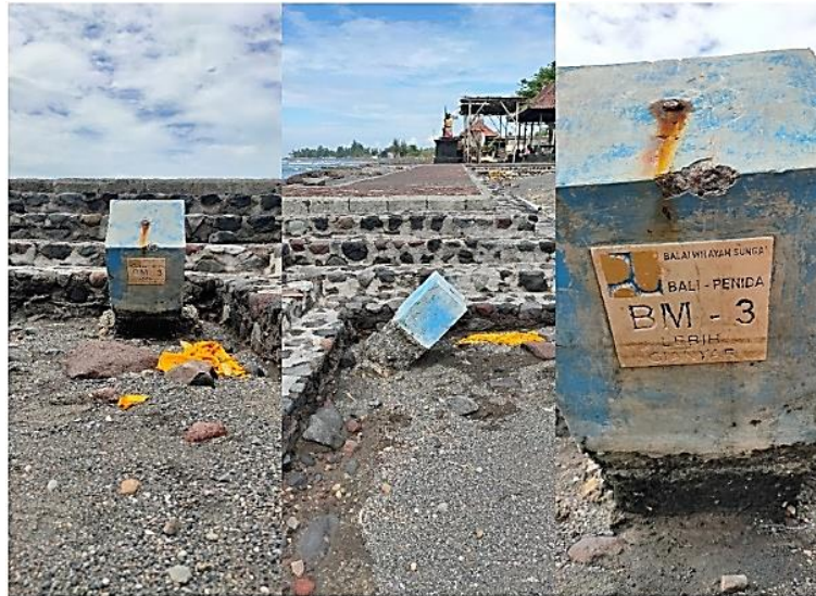
Figure 18. The Condition of the Bench Mark (BM) belonging to the Bali-Penida River Area had Collapsed due to Abrasion
